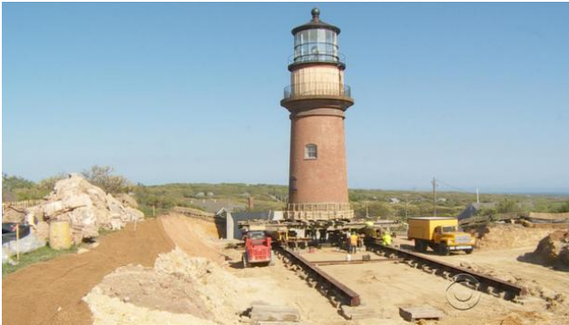
Crews work to move the Gay Head Lighthouse inland, away from the edge of an eroding cliff.
